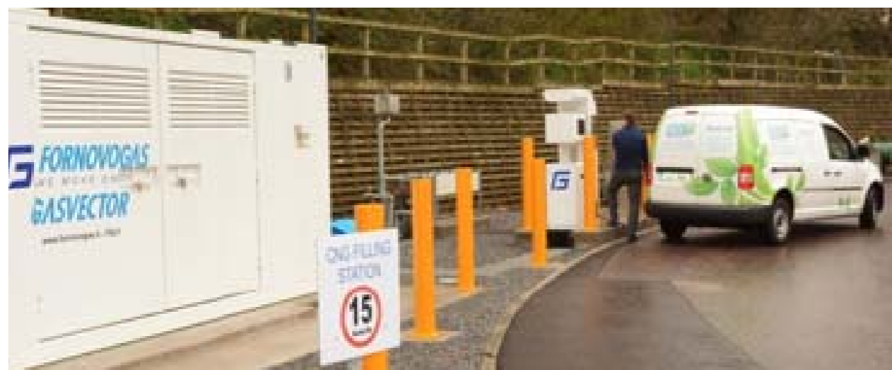
Figure 7 Gas Networks Ireland fast-fill station, Gasworks Road, Cork
