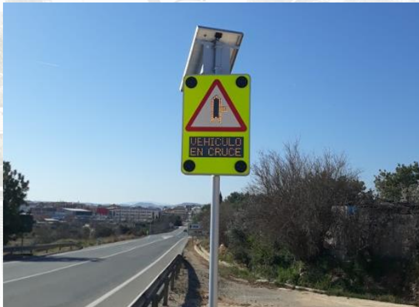
Illustration 49. Example of Smart Crossing in operation. Source: DGT
