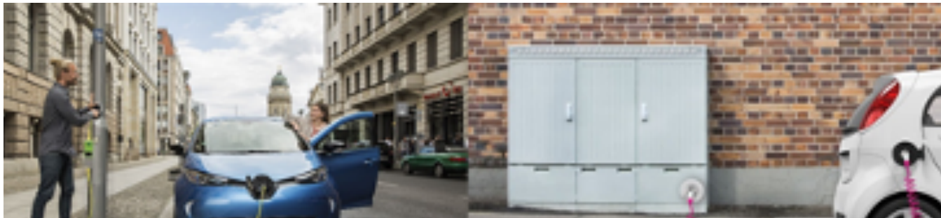
Figure 8: integration of recharging solution in a lamp post (left) and telecom distribution box (right)
