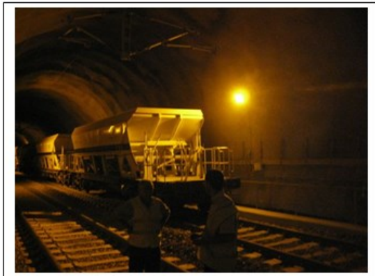
Inside the tunnel. The excavation and lining is fully complete as is the coating, waterproofing and drainage.
