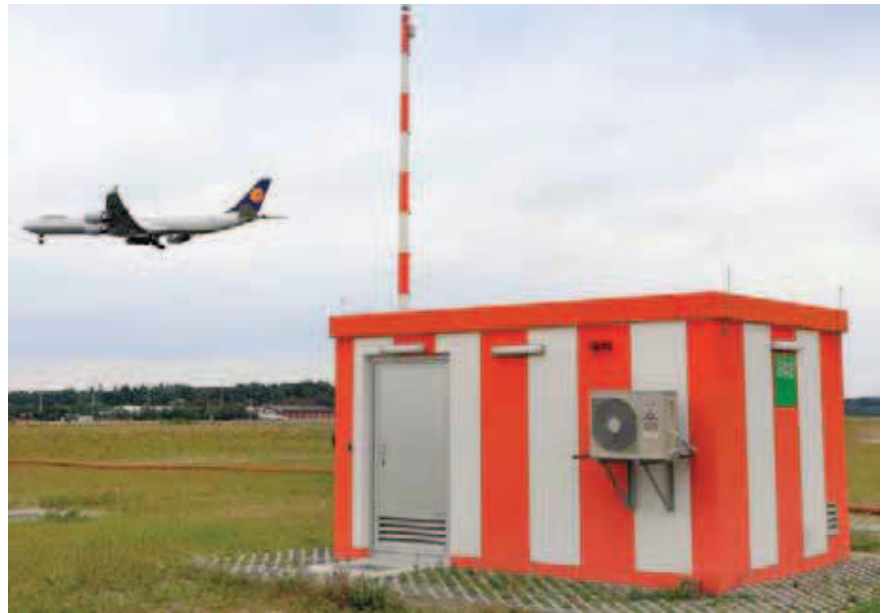
GBAS installation at FRA – Europe’s first hub to implement the Ground Based Augmentation System technology
